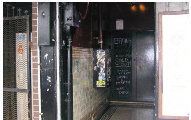
EXAMPLE OF POOR ENTRANCEWAY TO A NIGHTCLUB
