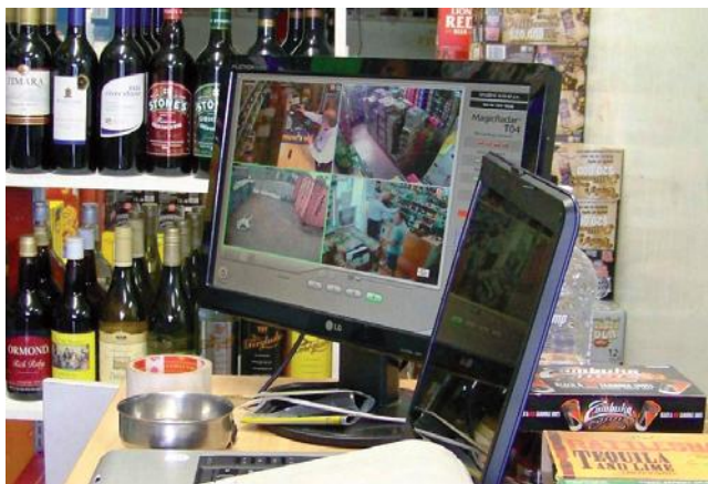
EXAMPLE OF CCTV MONITOR
