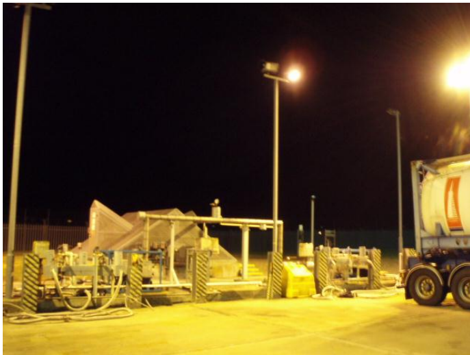
High pressure Sodium lamps in floodlights providing both operational as well as security lighting.
