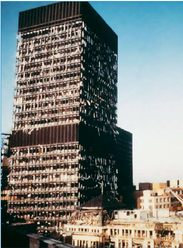
Figure 2-9 Blast damaged façade
